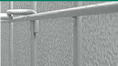
3.) Frost-free inner wall following the defrosting process
